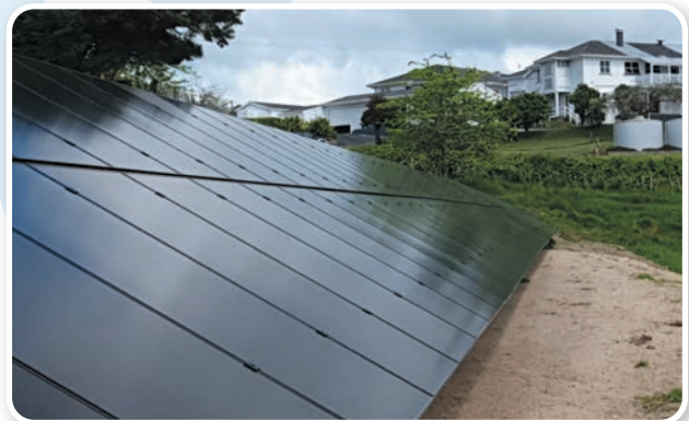
Hauora Hokianga's solar panels
